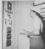
Marcial St. Jago is shown here taking a reading from the cat cracker substation switchgear box.
